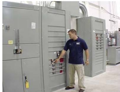
AC power entry at D.L.S. facility
